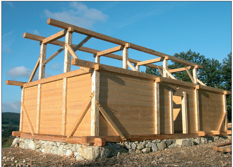
■ Fig. 9 Residential: Threshold construction with rectangular shaped beams, vertical bolt board walls and the substructure for the rafters. Note the supporting diagonal woods on the corners.
