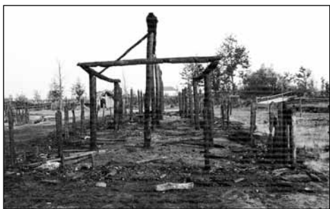
Fig. 7 Burnt-down Stein 29, seen from the northside June first 1995. The fire started on the right-corner. ■
